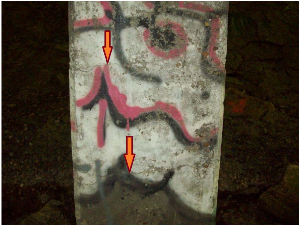
Figure 5-6 Route 1 over Hazel Run- horizontal cracks at Column 4, Pier 1 (38.28778, -77.48687).
