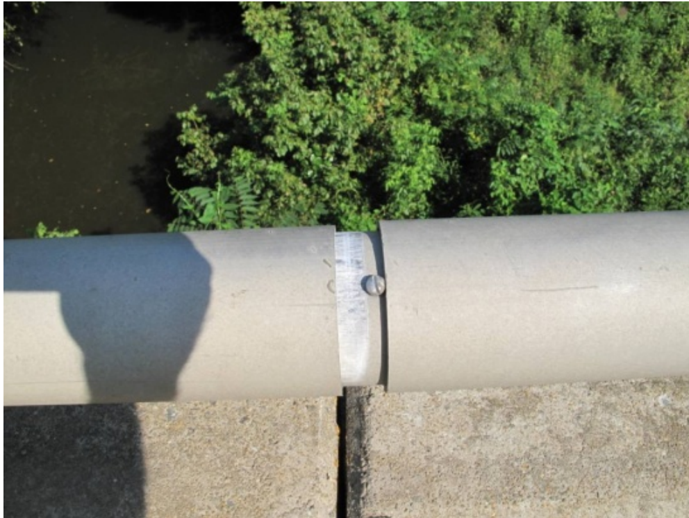
Figure 5-3 Courthouse Road over South Anna River - displacement of railing (37.98064, -78.04818).
